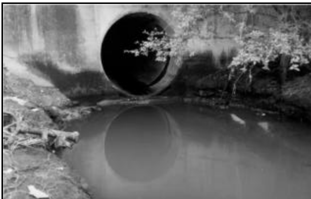
Oil contamination at Tucks Rd drain
