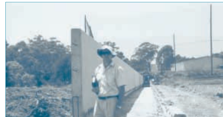
The Sierra Place flood retarding basin on Upper Toongabbie Creek at West Baulkham Hills was raised by 2.5 metres to enlarge the capacity of the basin.
