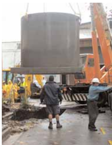
As part of the WSUD Capacity Building Program, participants at one of the seminars visited Rockdale Council installing an underground tank to store rainwater for non-potable uses in the Council building.
