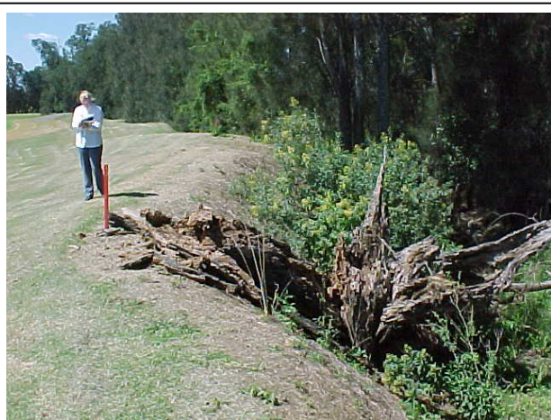
Typical decay of willow trunks, Greystanes Creek
