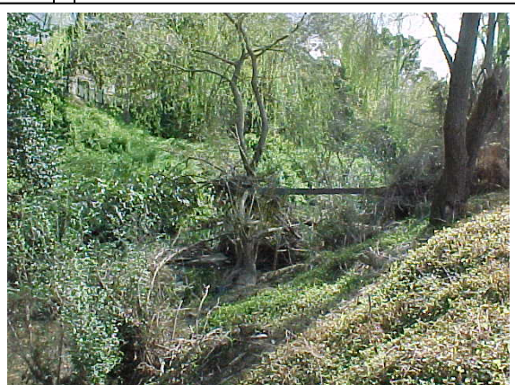
Channel constrictions and sedimentation caused by willows, Speers Rd, Darling Mills Creek, Northmead.
